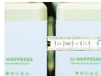
Fig. 5-14: 10 mm clearance between the batteries
